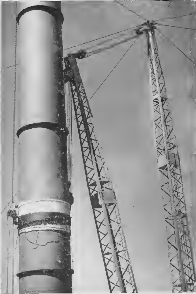
WELDER LAMPE climbs aloft, cuts lashings after lift. WELDER LAMPE ta subi na laria, pa corta cablanan.
